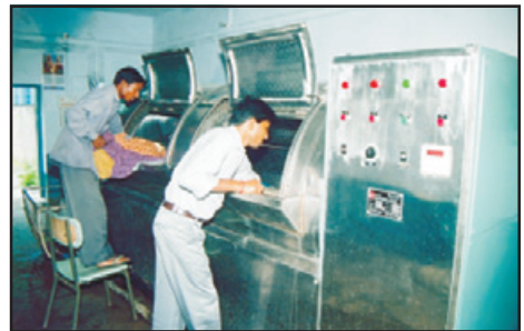
Mechanised laundry at RINPAS Jharkand
